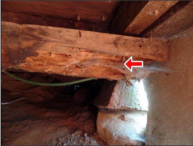
4.2 Item 1(Picture) Wood destroying insect damage
