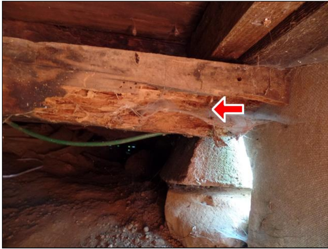
4.2 Item 1(Picture) Wood destroying insect damage
